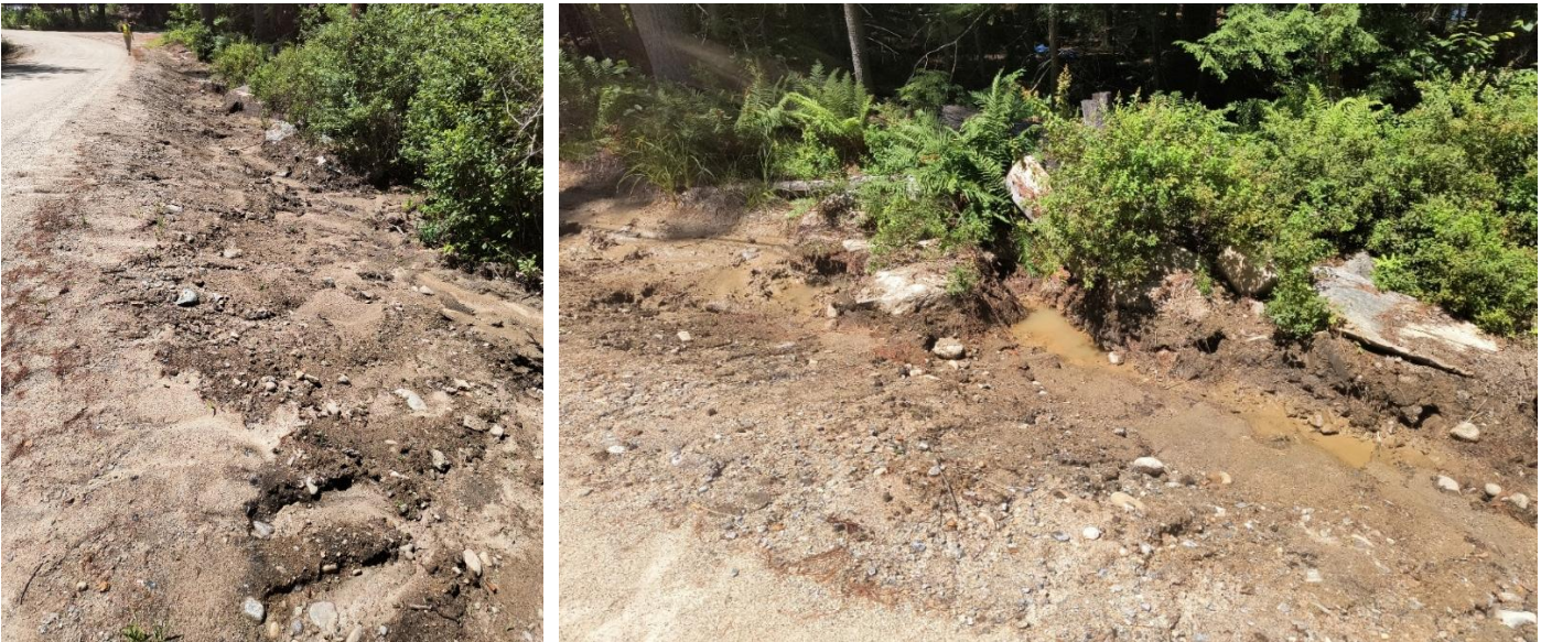
Scouring on road shoulder (left) leads to a large, disturbed area with sediment built up (right).
