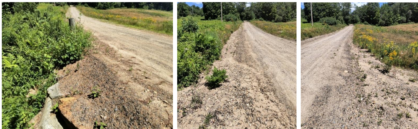
Culvert at bottom of hills (left) and gullies along ditch (middle and right).
