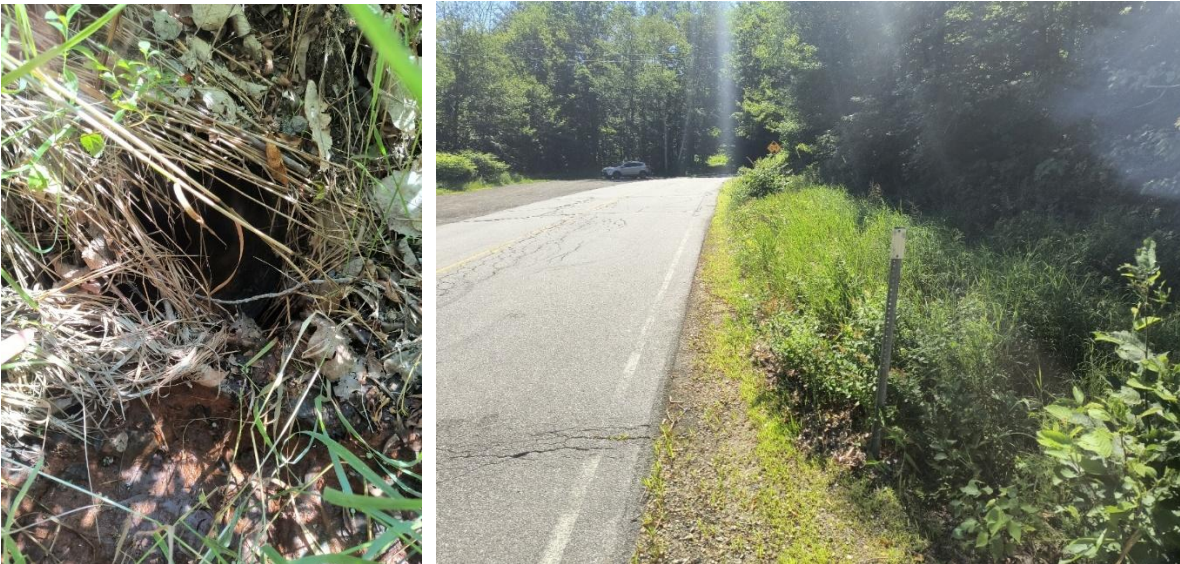
Partially clogged culvert (left) that drains vegetated swale (right).
