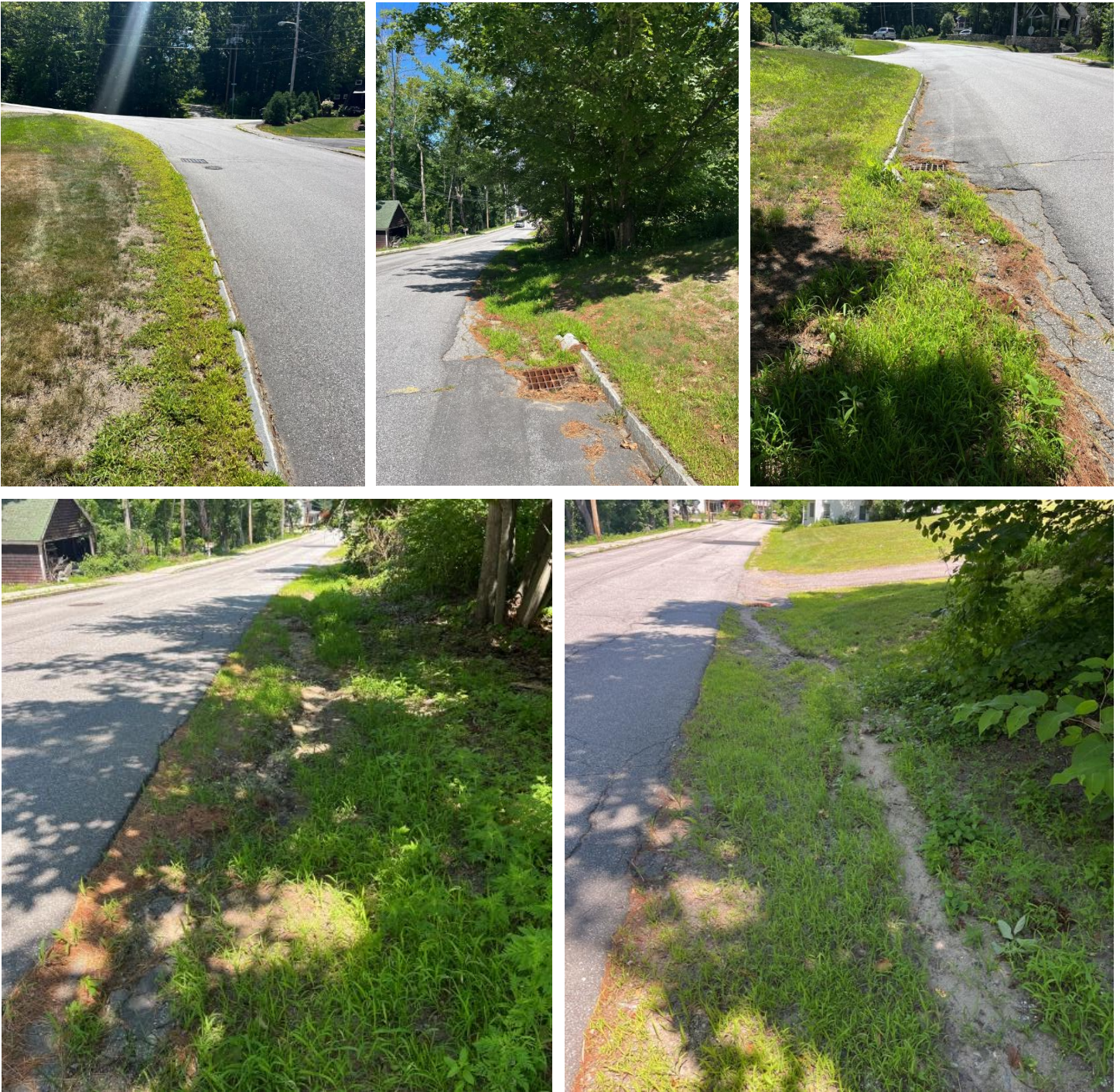
Catch basins on the street (top left, middle, and right) and erosion gullies on road shoulder (bottom left and right).
