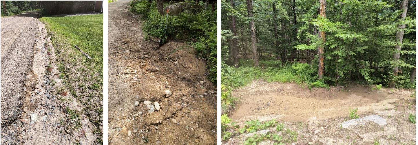
Gullies and erosion along road shoulder (left and middle) that lead to sediment deposits (right).
