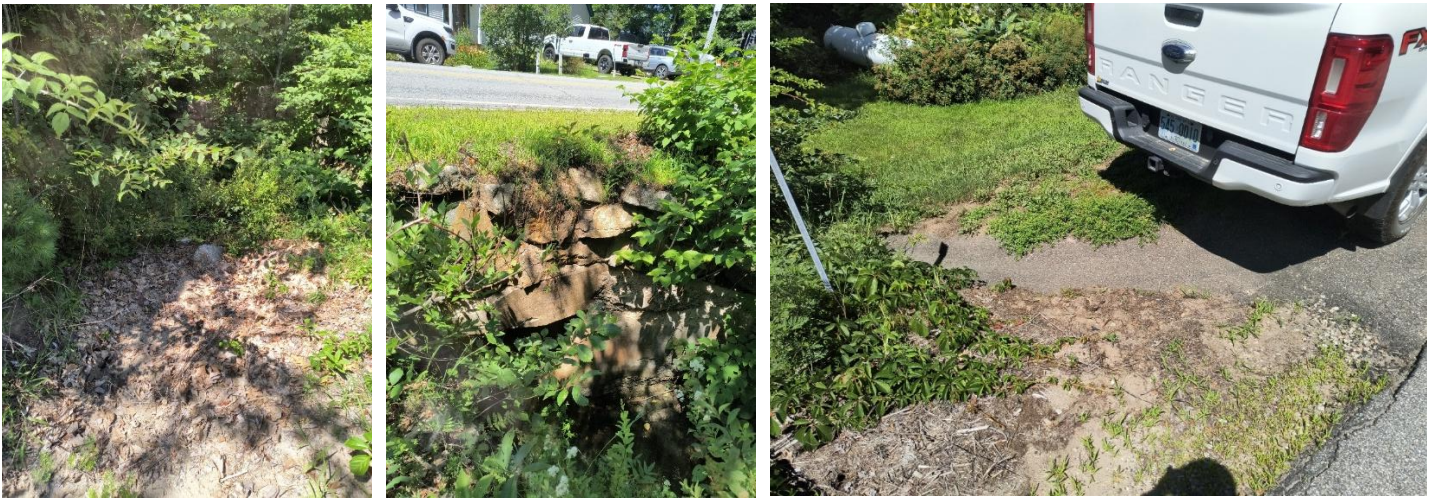
Sediment buildup at end of gully that transports to stream (left). Lack of vegetation at culvert inlet (middle). Paved swale on downstream side that directs stormwater to stream (right).
