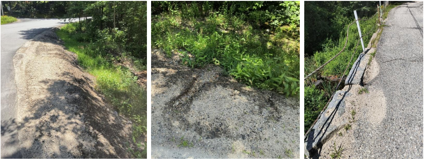
Loose asphalt material on road shoulder with some small gullies (left and middle). Sediment buildup on bridge (right).
