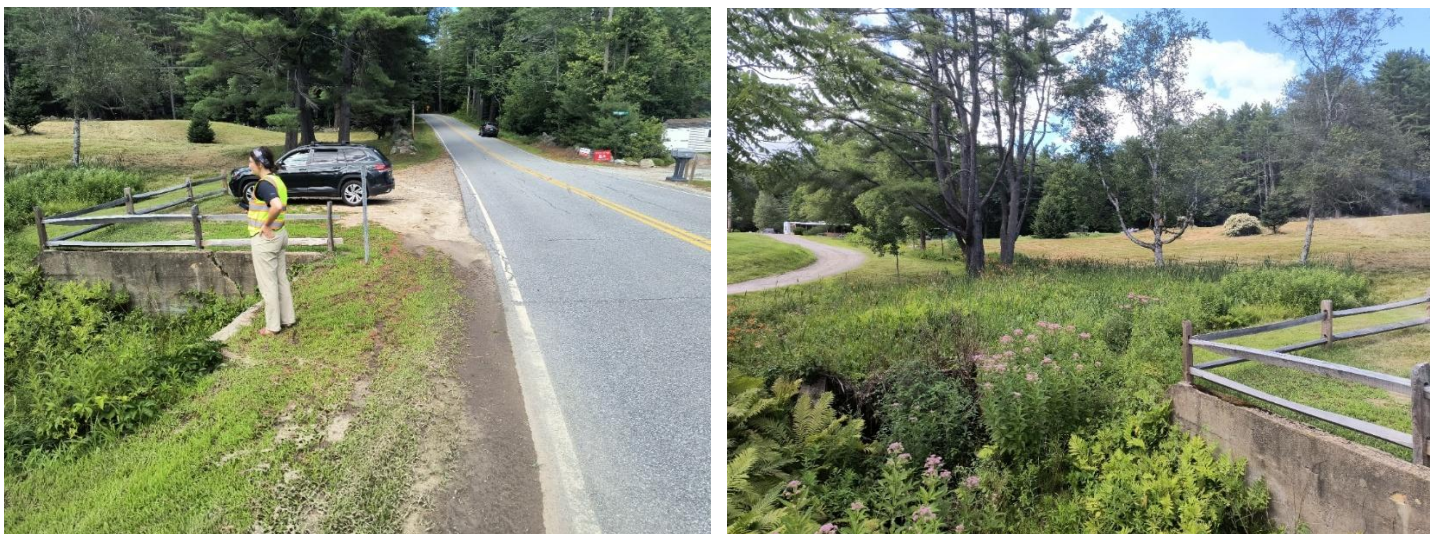
Culvert inlet with lack of vegetation (left) and upstream with narrow buffer through campground (right).
