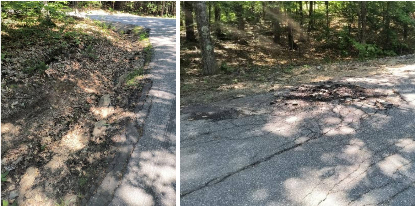
Erosion in the road ditch of the island (left). Road surface erosion (right).
