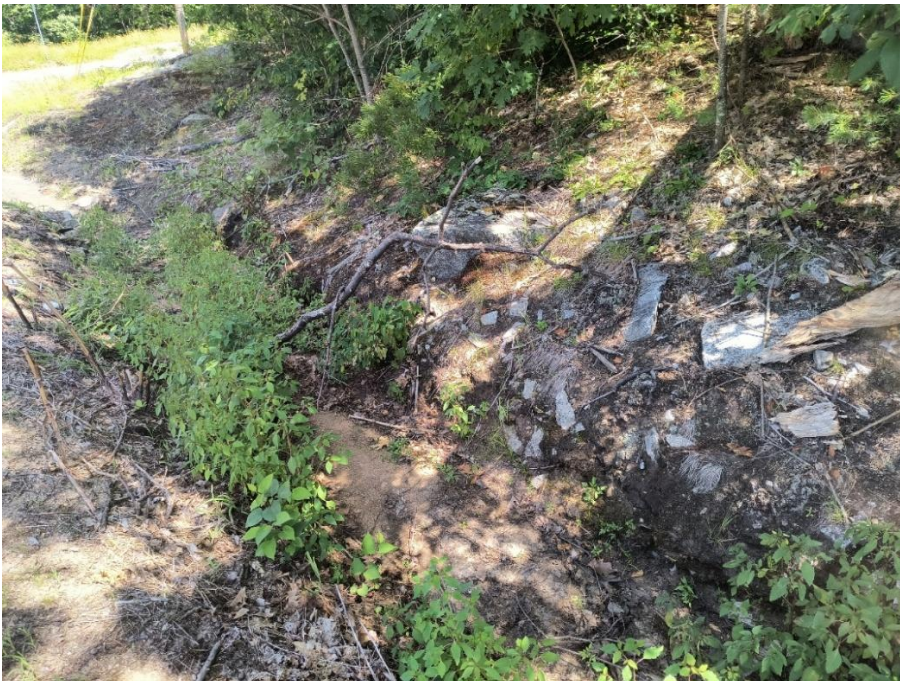
Erosion of ditch and bank with evidence of sediment transport.
