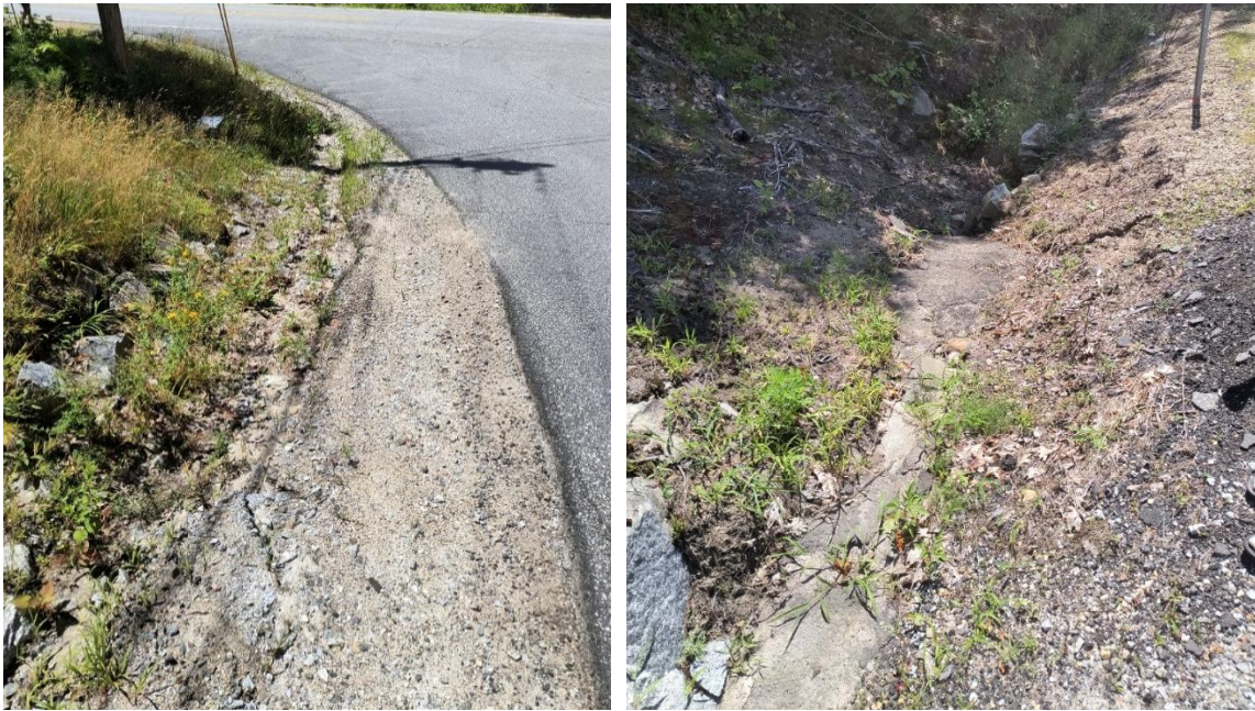
Eroding road shoulder (left) which leads to a paved swale and culvert (right).
