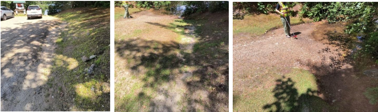
Large sandy parking lot (top left) leading to boat ramp which has some erosion (top right and bottom right). A gully along parking lot (bottom left) leads to boat ramp (bottom middle).
