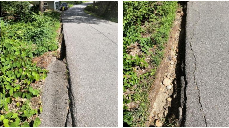
Paved swale on road shoulder (left) that creates a gully downstream (right).
