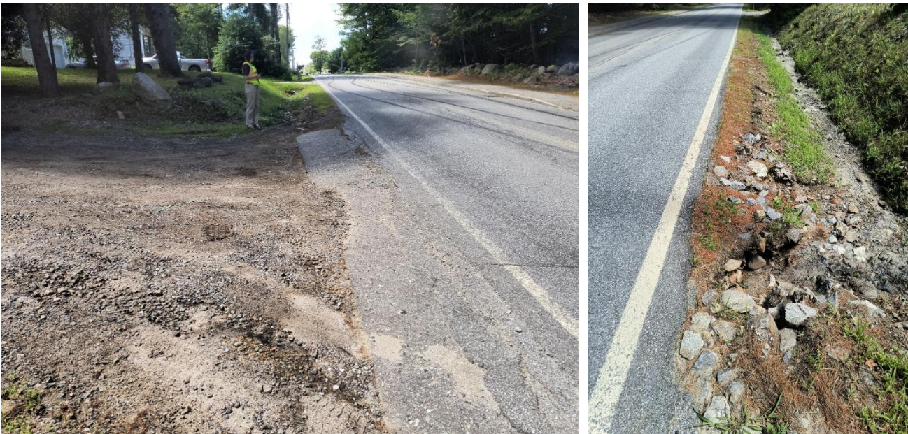
A commercial driveway is eroding and transporting sediment (left) to the downstream ditch, causing erosion and sediment build-up (right).
