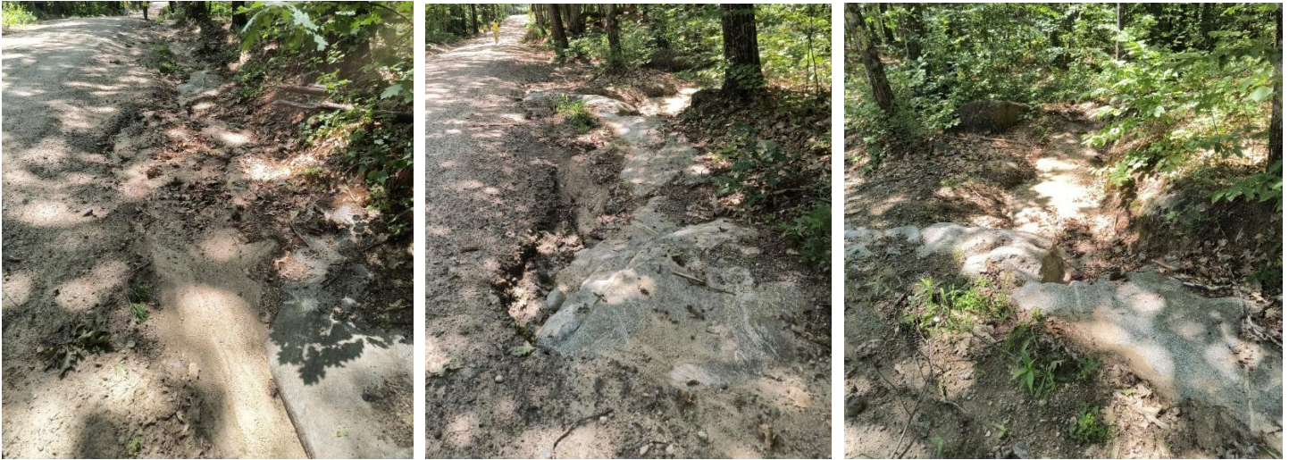
Erosion and sediment build-up in ditches (left and middle) leading to turnouts into woods (right).
