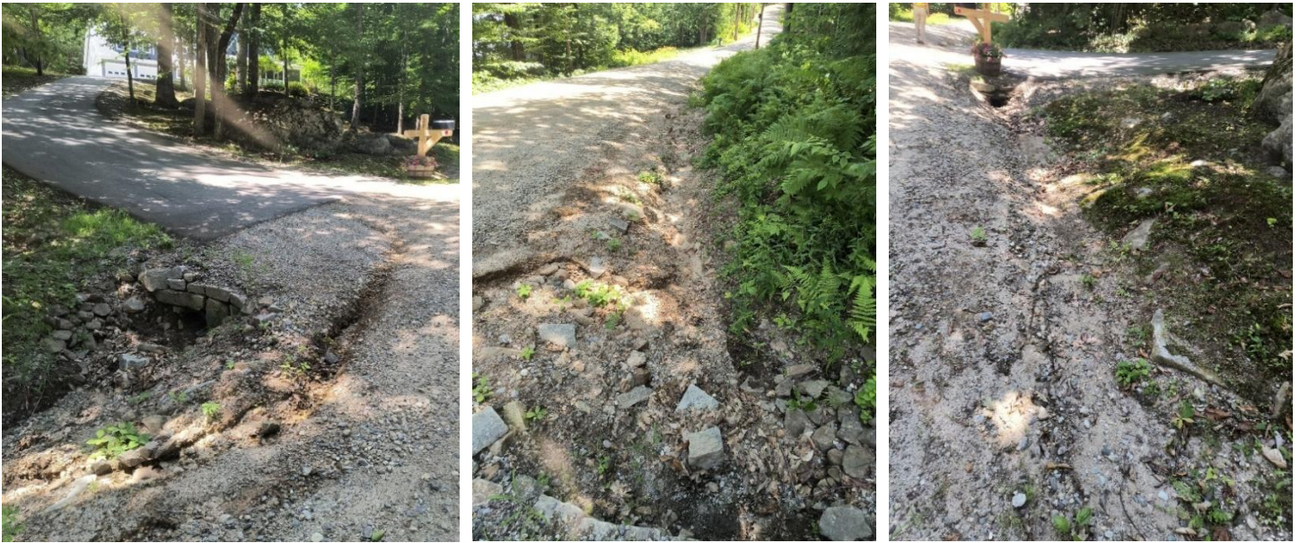
Gullies along bottom of driveway (left) lead to ditch erosion and sediment transport (middle and right).
