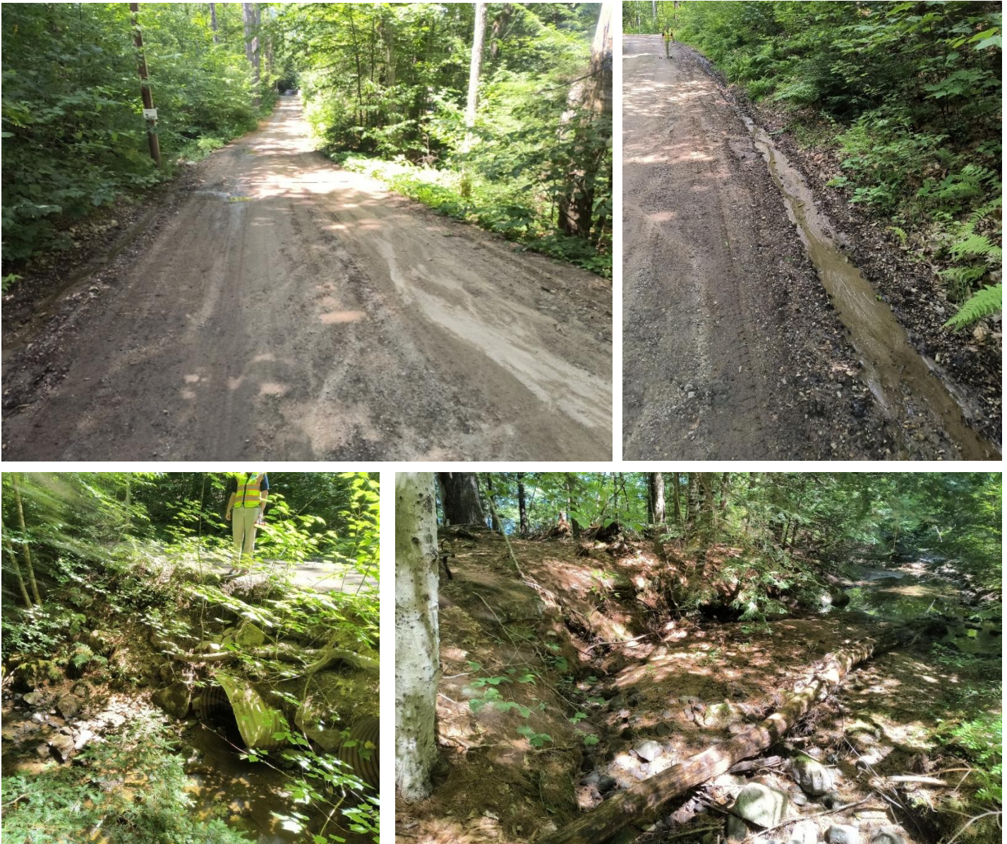
Gullies on road surface and shoulder (top left and top right) lead to outlet of a double culvert (bottom left) and a stream that leads directly to the lake (bottom right).
