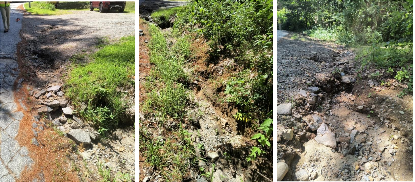
Gully beginning on the driveway of 2 Pollard Shores Road (left) and continuing down the road (middle and right).
