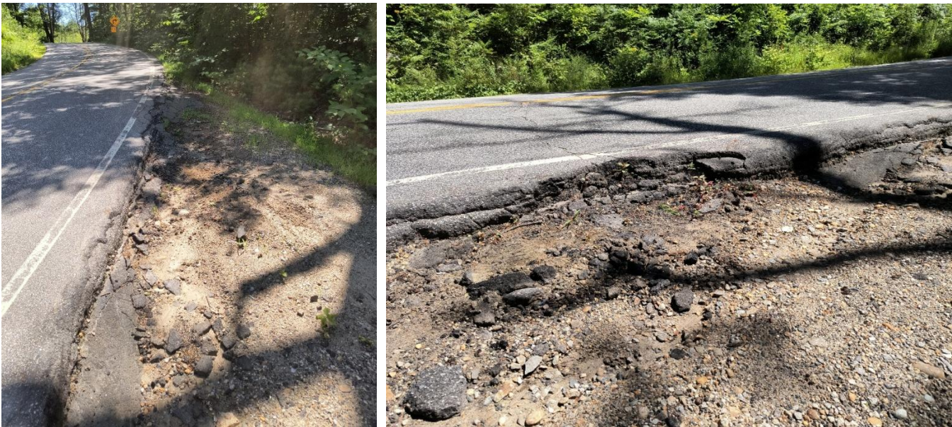
Eroding road shoulder and parking area (left and right).
