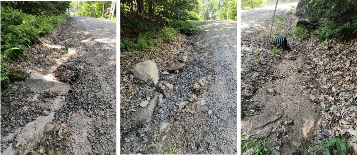
Washed out check dams caused gullies to form in ditch (left and middle) leading to sediment buildup at the culvert inlet (right).
