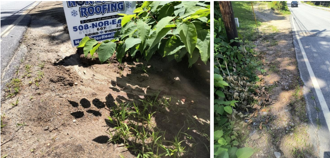
Road shoulder/ditch erosion and sediment transport (left and right).
