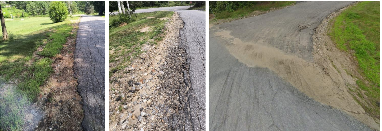
Roadside erosion (left) that becomes wider further down the road (middle) and deposits sediment at the intersection (right).
