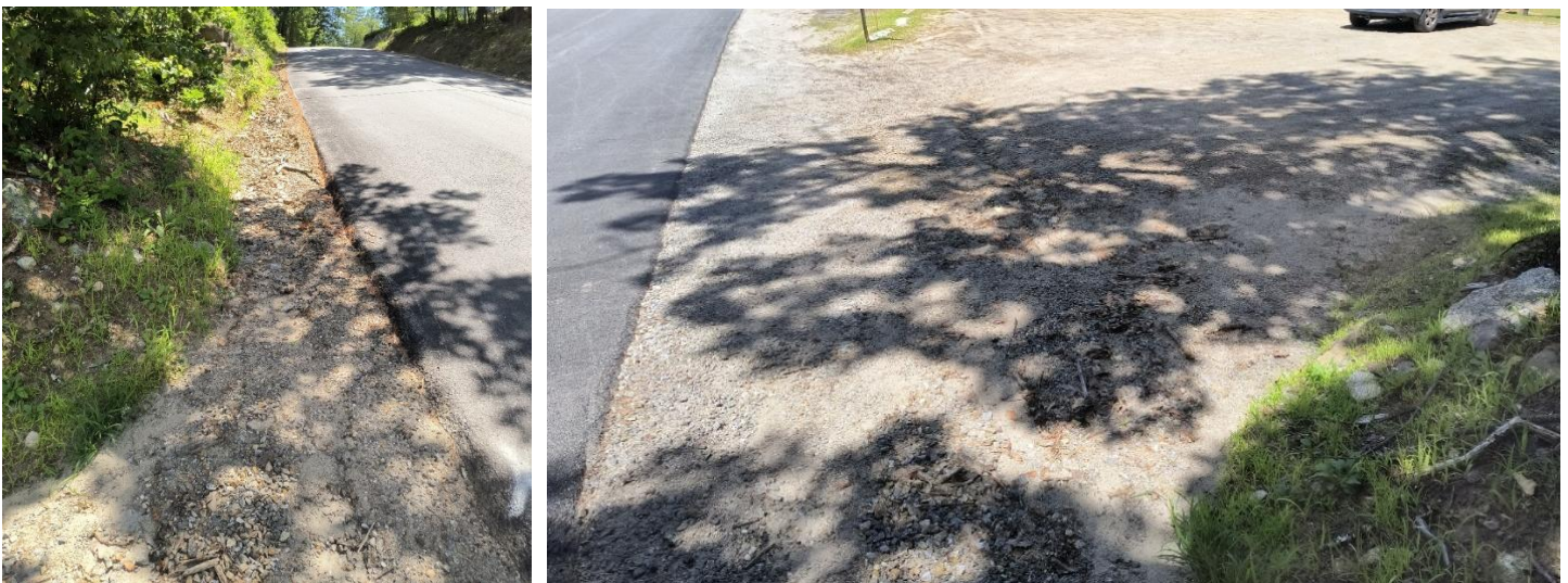
Gully along edge of road (left) leading to more gullies in parking lot (right).
