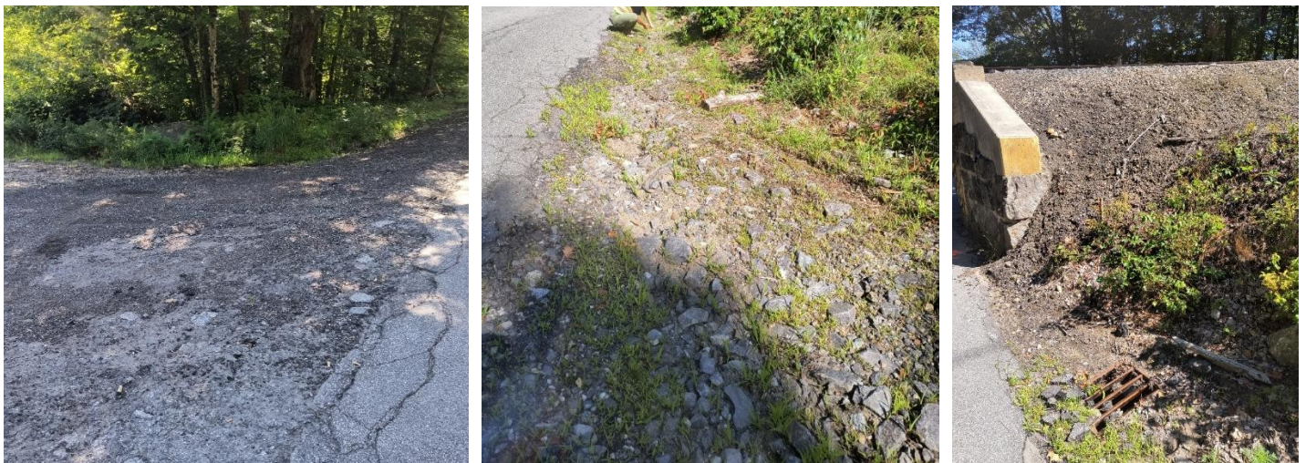
Loose asphalt parking area (left) uphill of a gully (middle) that leads to a clogged catch basin by the railroad bank (right).
