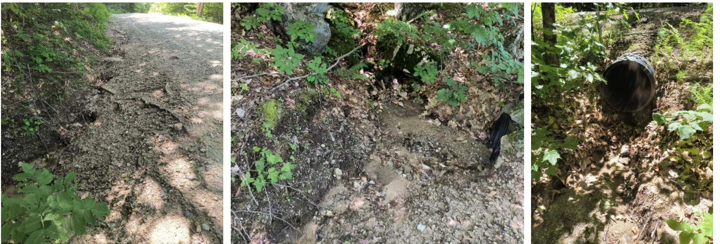
Sediment transport to culvert inlet (left) with lack of buffer and sediment accumulation (middle). Culvert outlet is perched and sediment deposit is visible (right).
