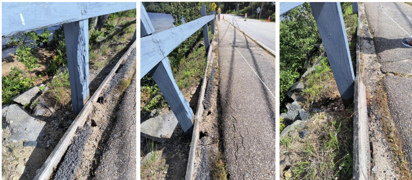
Eroding edge of sidewalk with sand accumulation and bare soils (left, middle, and right).
