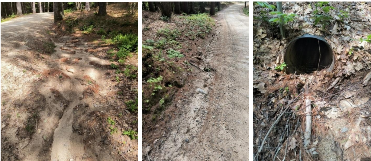
Road shoulder/ditch erosion and sediment transport (left and middle) leading to culvert that is partially filled with sediment (right).
