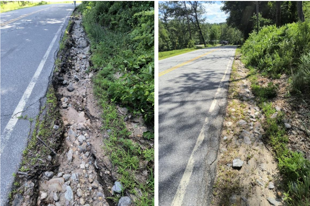
A gully has formed in the road shoulder (left), which is filled with sediment (right).
