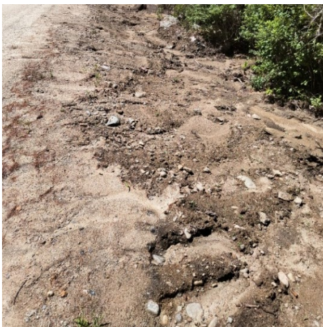
Large disturbed area with sediment built up (top) and scouring on the road shoulder (bottom).
