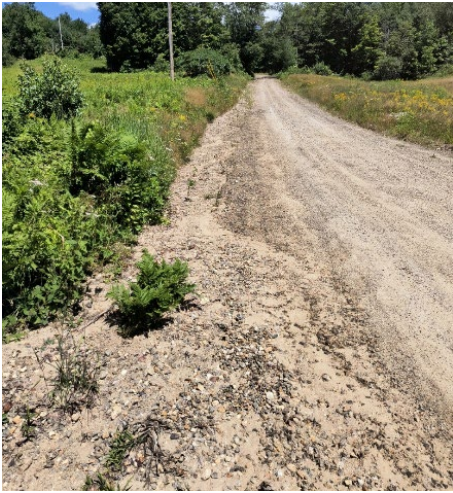
Large gully along the road shoulder.
