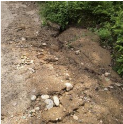
Sediment deposits in the forest (top) and road shoulder erosion (bottom).
