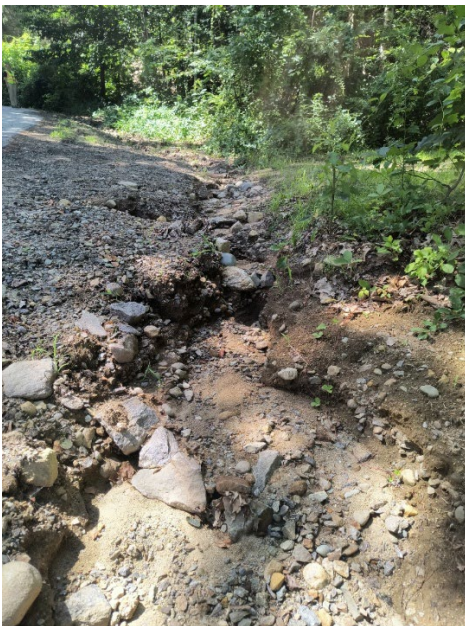
Large gully beginning at 2 Pollard Shores Road.
